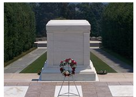
The crack can be seen underneath the words "An American" and above the word "Soldier."
