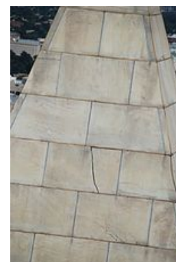
Crack in a stone at the top of the monument after the 2011 Virginia earthquake
