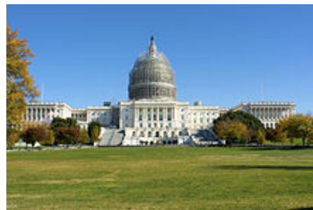
The United States Capitol, with scaffolding erected to facilitate restoration work on the dome (November 2014 view)
